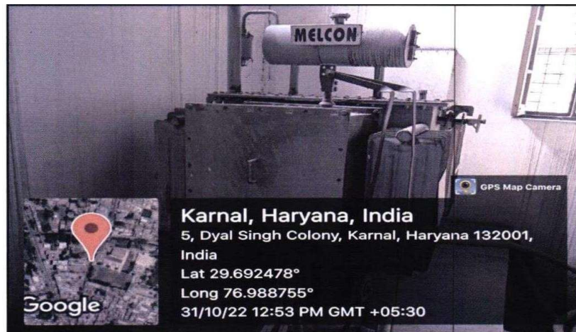
Image of 200kVA transformer
