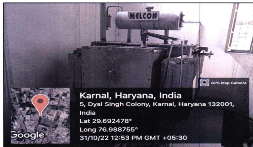
Image of 200kVA Transformer
