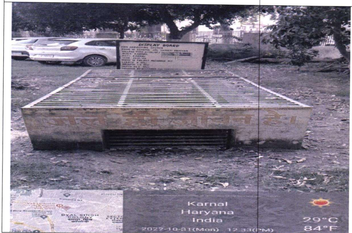
Rain Water Storage Tank
